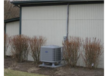
Heat pump for new HVAC
