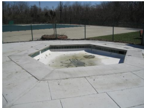
Baby Pool Repair Complete: New Coping, Drains, Tile, & Depth Markers (the plaster is not complete in this picture)
