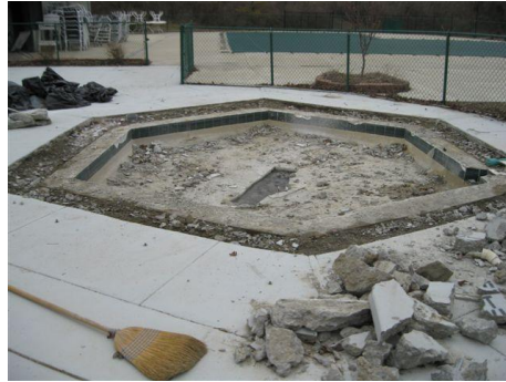
An "in process" picture of the Baby Pool Repair & Compliance with VGB
